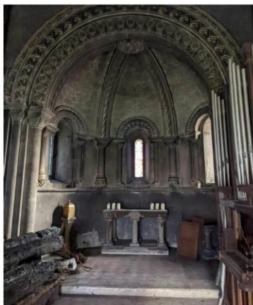
Sanctuary with Smoke Damage
