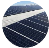
Solar PV Panels
