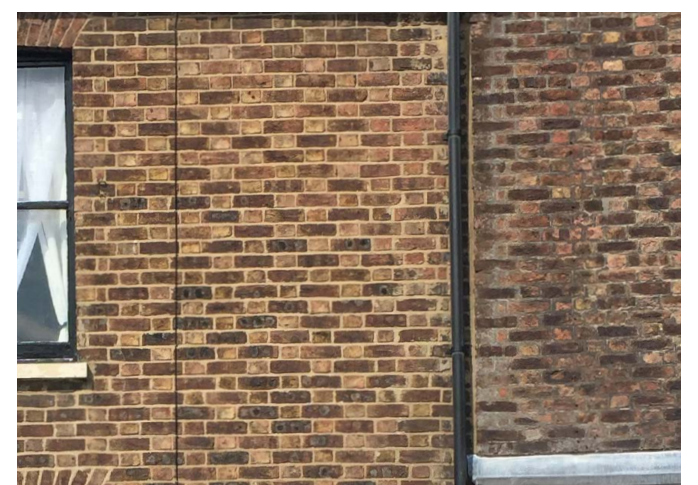
Photograph of 'speckled' brickwork in King's Lynn
