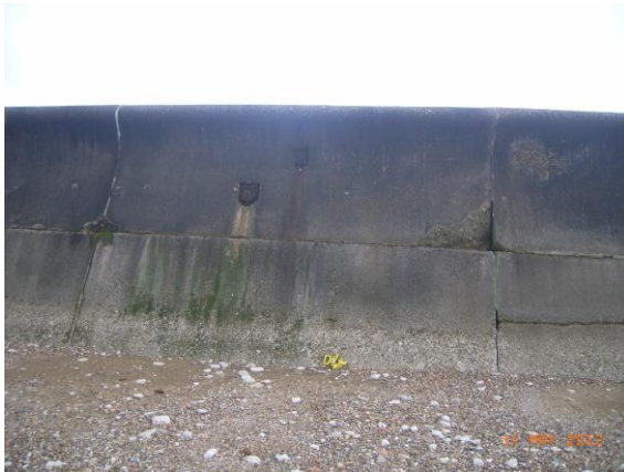
Figure 13-2 Section G seawall panel with cracking at joints and loss of concrete
