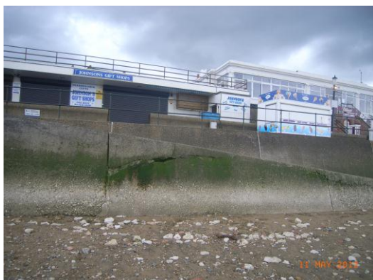
Figure 12-2 Crack at seawall panel 3.
