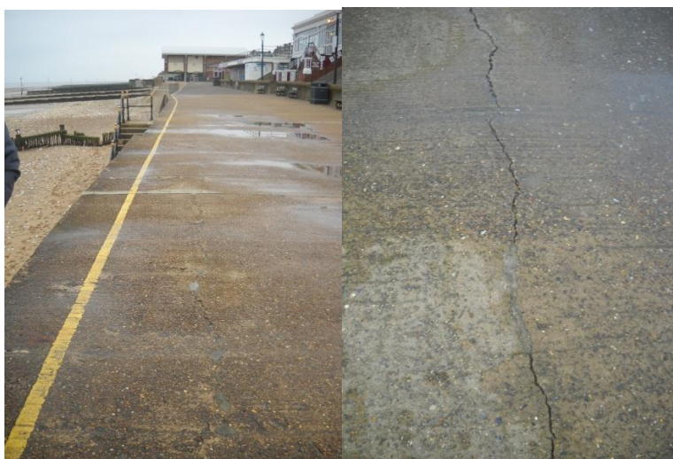
Figure 11-3 35.4m long crack spanning between planes 37 to 43
