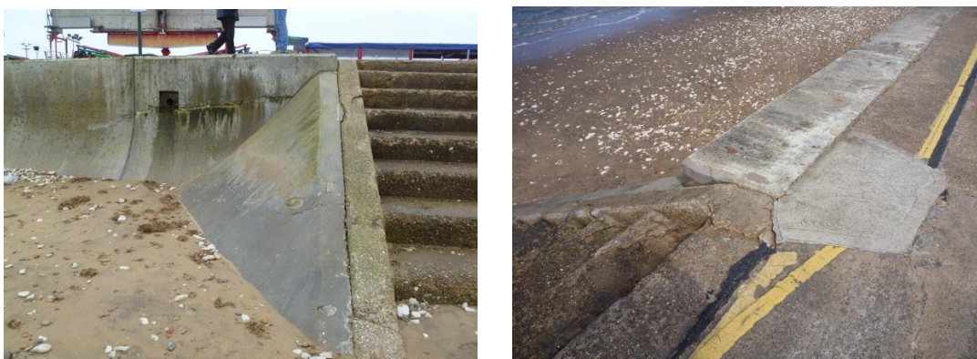
Figure 8-2 Section B, large crack observed in panel 1
