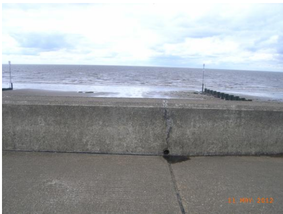
Figure 13-3 Recurve wave wall upstand with cracking at an outlet point
