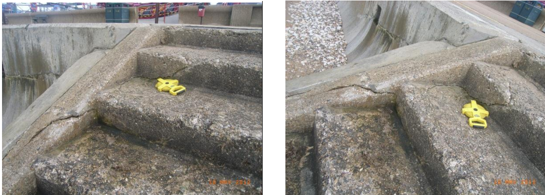
Figure 7-2 Significant crack across the seawall panel 68 of the Section A
