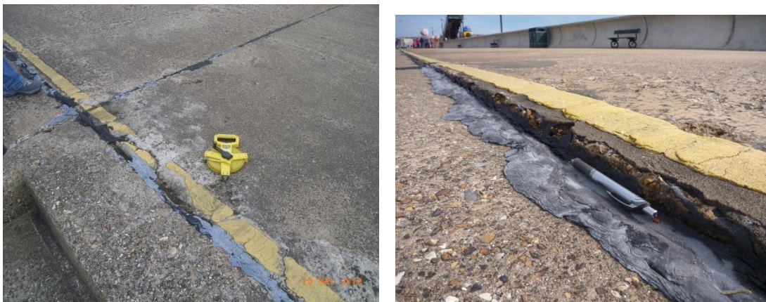
Figure 7-3 Panel 64 cracking and sealant loss (left) and 40mm settlement (right)
