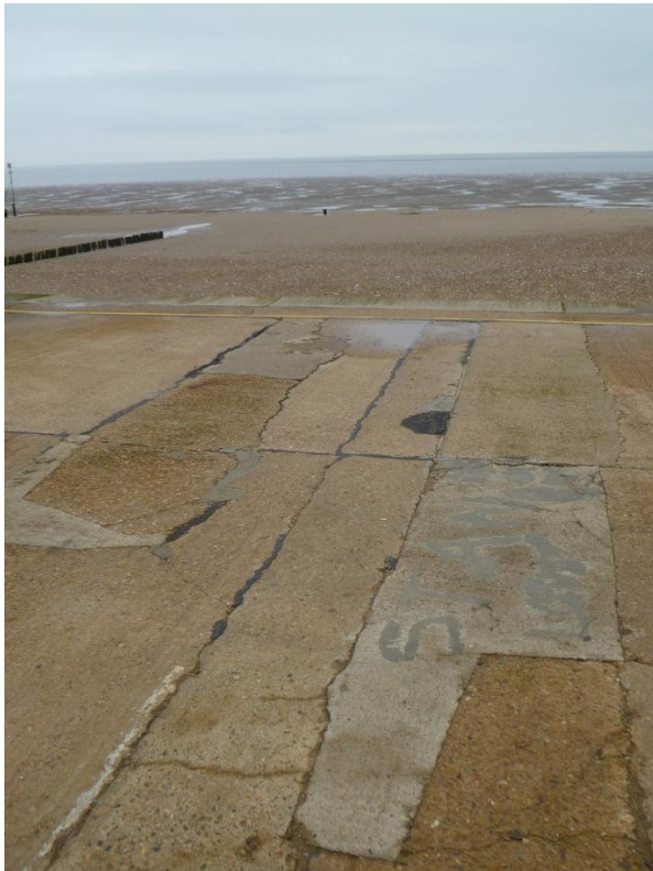
Figure 9-2 Promenade slab with heavy patch repairs
