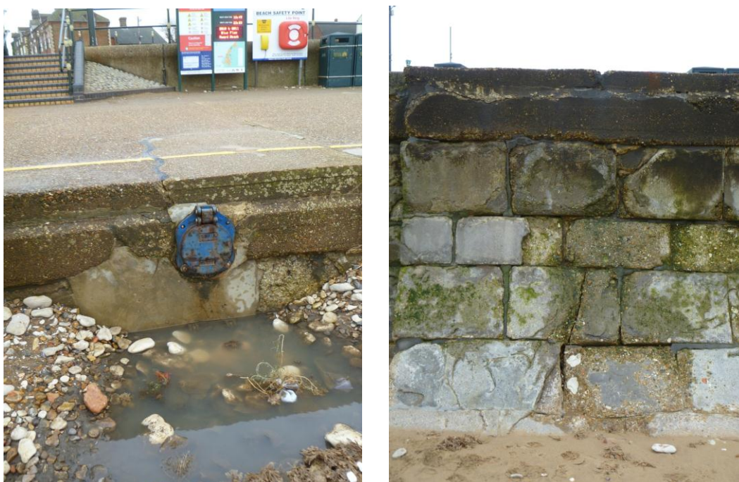
Figure 11-2 Outfall at panel 5 and seawall panel in poor condition (left), typical seawall panel condition (right)
